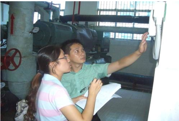
检测龙岗区检察院机房设备
